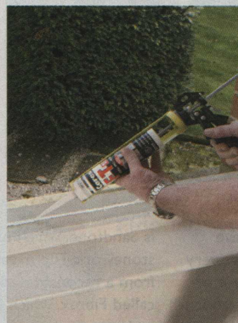
To resist driving rain under the new sill a bead of sealant is applied.
